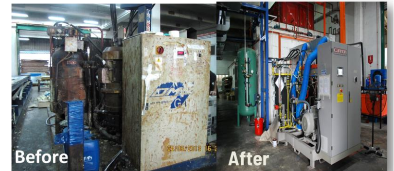
Technology conversion from HCFC-141B to Hydrocarbon (Cyclopentane)
